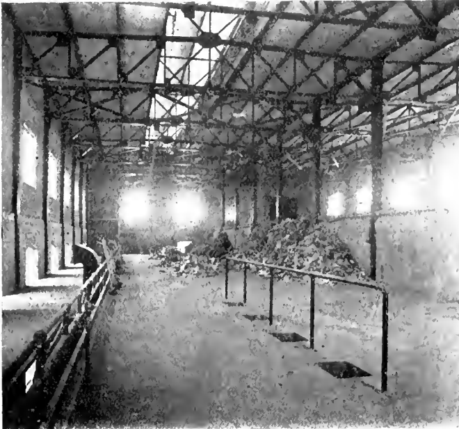
Garbage is dumped from tipping floor on right to charging floor and is charged into the furnaces through chutes.
